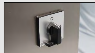
IMG. 6: Main power switch
