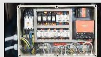
IMG. 4: Sealed electric box
